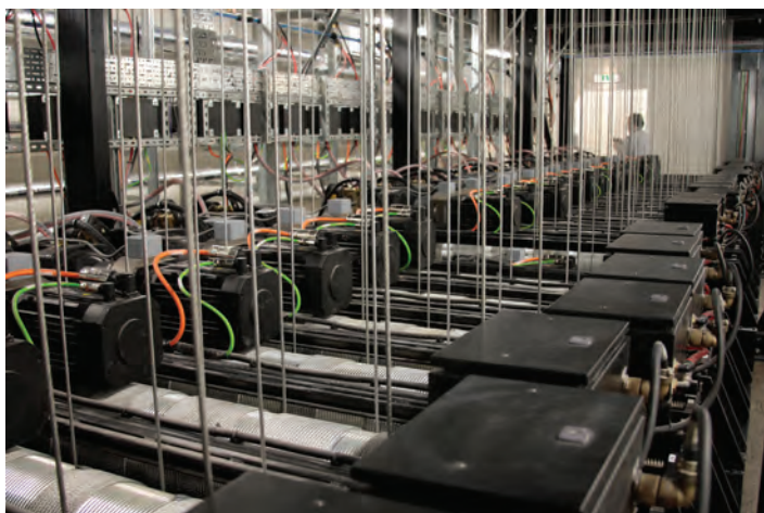
Stage Technologies' Big Tow winches in the machine room.
