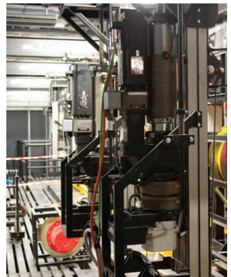
Detail of the machine room
