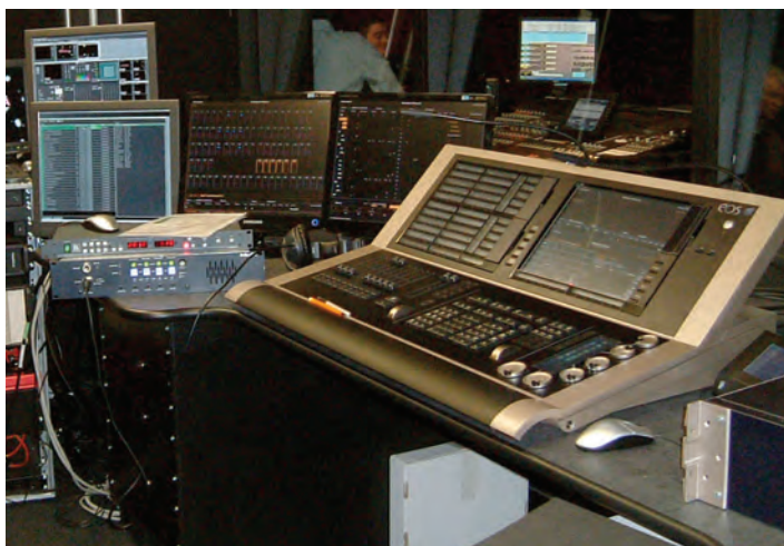
The ETC Eos lighting control system.
