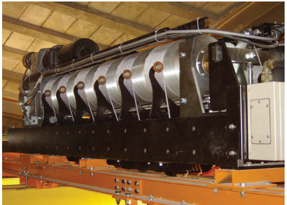
A BigTow 2 winch as installed at the Royal Festival Hall.
